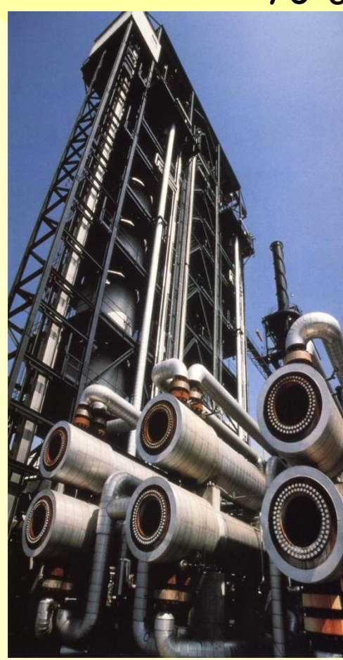
Hydrocracking unit Source: www.cevron.com
