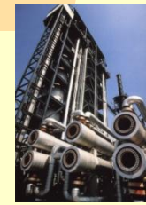
Hydrocracking unit Source: www.cevron.com
