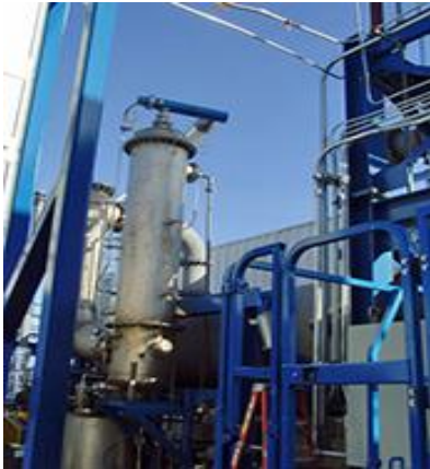
Gasification unit for syngas production
